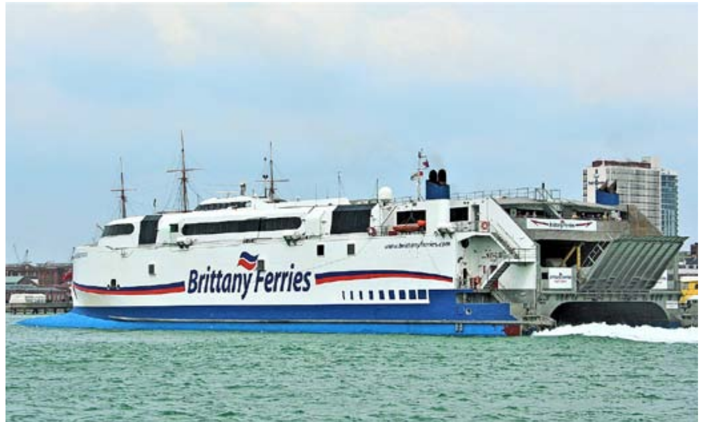
» This week FastCat ferry Condor Voyager arrived for the installation of a bow thruster. Her voyage from Ro-Ro berth number three at Poole Ferry Terminal to Falmouth took five hours. She sailed from Studland Bay to Falmouth Bay, a distance of 140 nautical miles, at an average of 28 knots. Condor Voyager is owned by Brittany Ferries who ran her between Portsmouth and Le Havre as Normandie Express. She was taken on charter by Condor Marine Services in June last year
